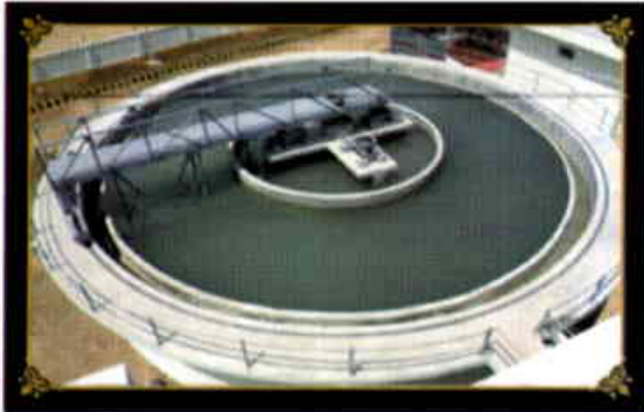
Rapid Sand Filters 59 mld capacity at Panagal of Nalgonda District Clarifloculator
