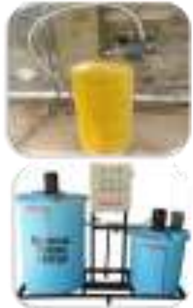
Chlorination based Disinfection System
