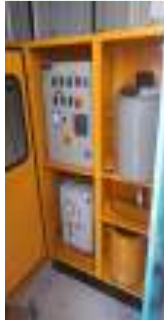
Electrochlorinator system for ground water
