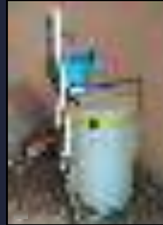
Electric liquid chlorine dosing pump
