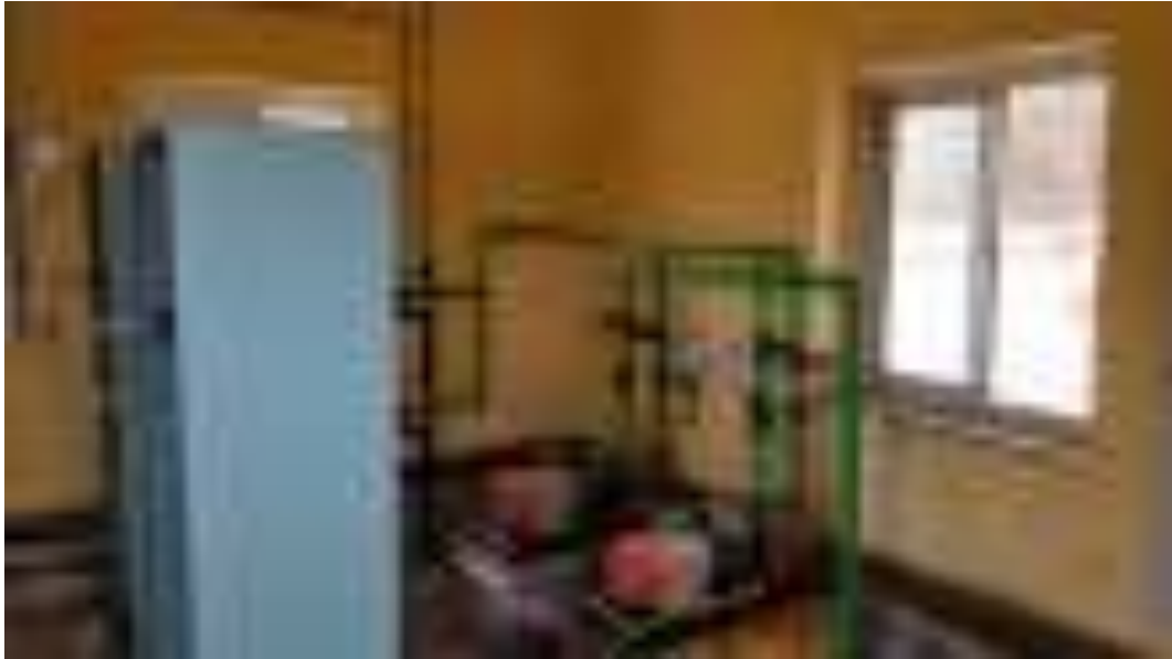
Chlorination by Electrochlorinator
