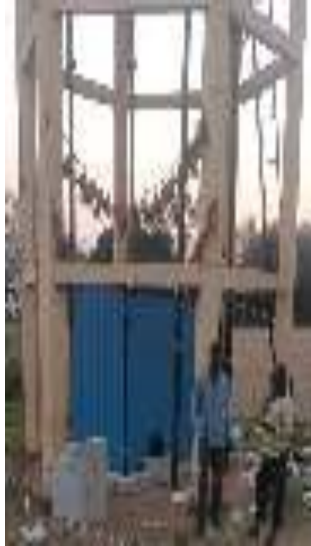
Chlorinator housing under OHT connected ground water
