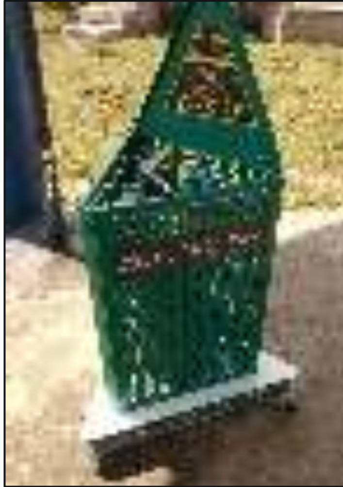
HiSafe Chloritron device in Pachama, Nasrullaganj, MP
