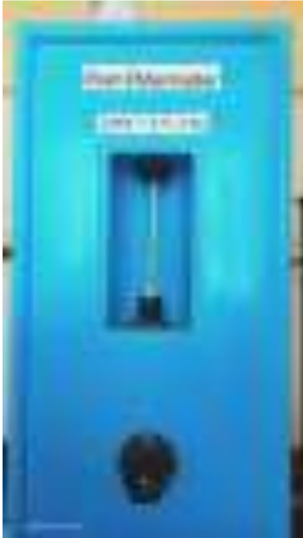
Post Chlorinator at MVS
