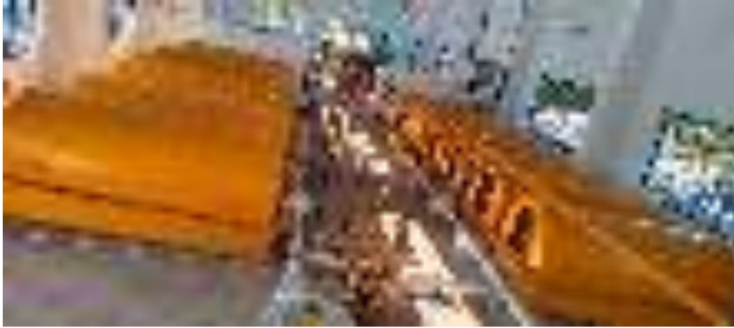
Gas Chlorination equipment at Raghavapur WTP
