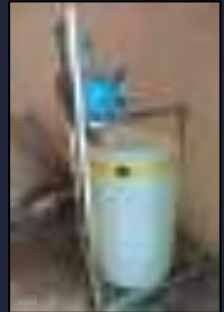
Electric liquid chlorine dosing pump
