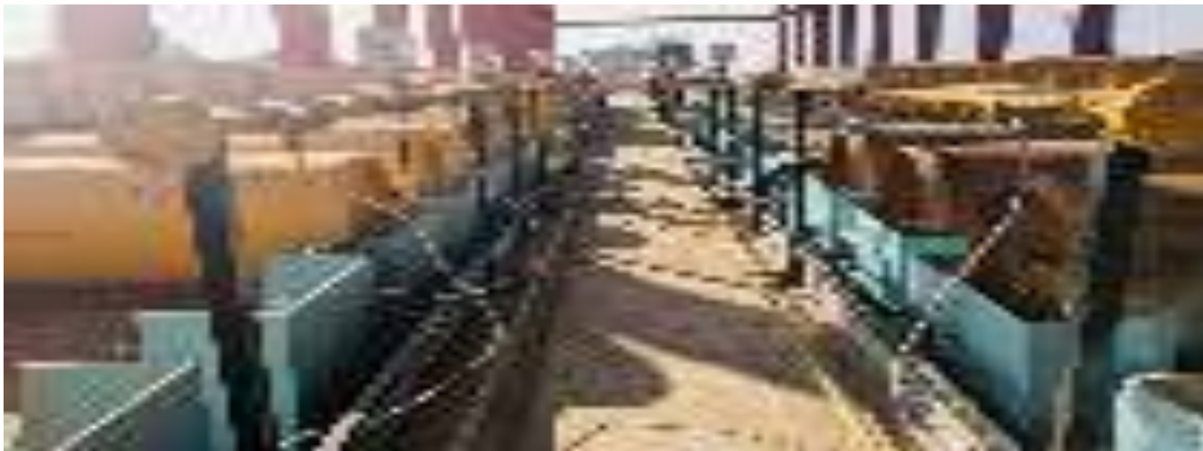
Chlorination by Chlorine Gas Cylinder at WTP Surajpura
