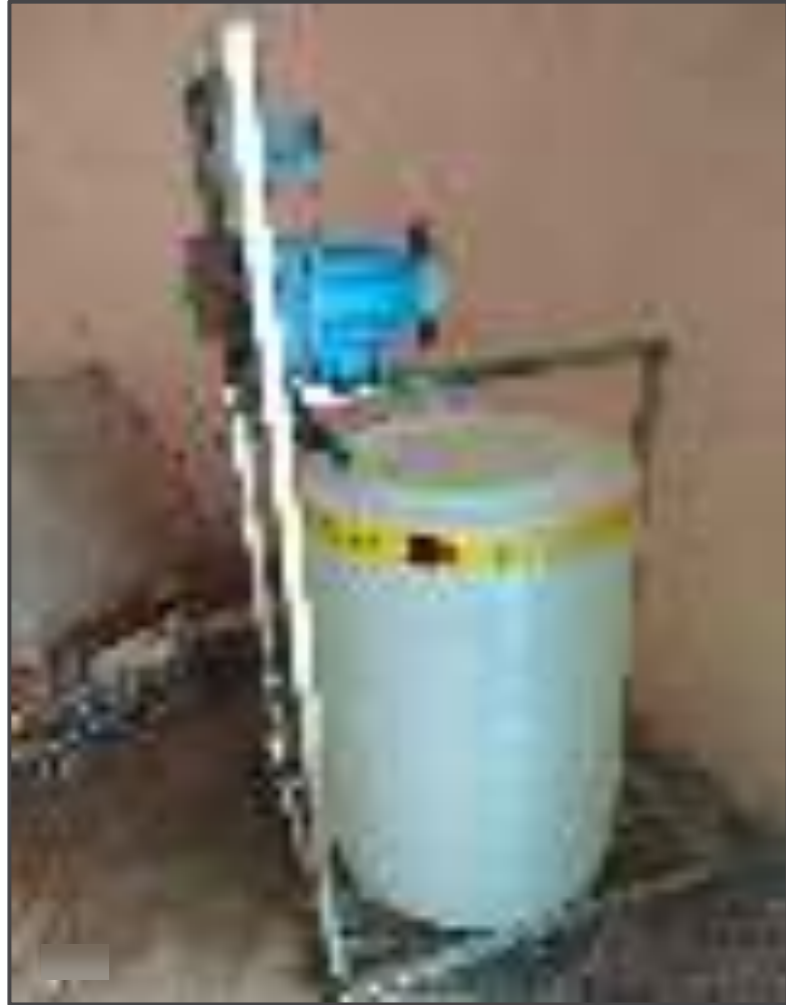
AC 6 Mechanical Dosing pump device in Kanhasiya, Fanda, MP
