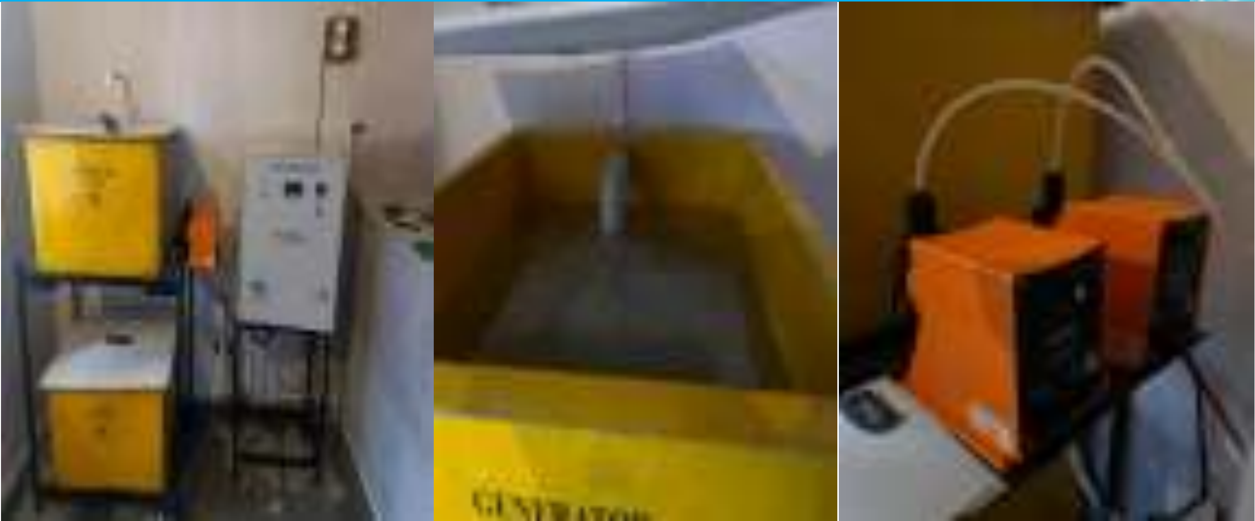
Chlorination through Nacl (salt) in the Ulihatu water supply scheme, Khunti District
